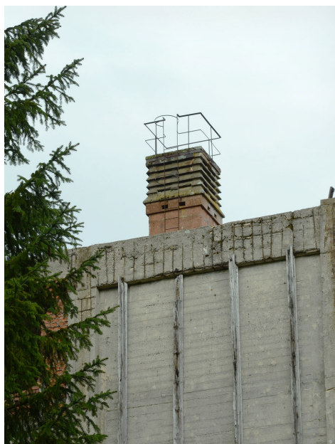
Smokestack and processing plant facade. Construction made of reinforced concrete was covered by insulating wooden layer.
