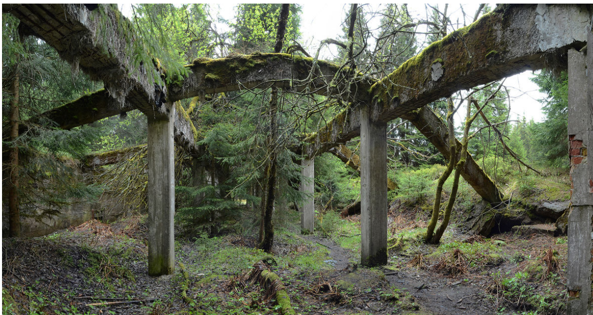
View in the processed ore warehouse; remains of roofing and reed isolation are visible on the ferroconcrete frame.
